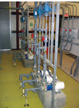
The containment remedy at Lowry Landfill consists of multiple components and state-of-the-art technologies.
