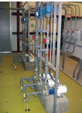
The containment remedy at Lowry Landfill consists of multiple components and state-of-the-art technologies.
